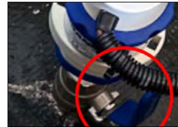
1100 GPH Fill Pump Valve Handle.
