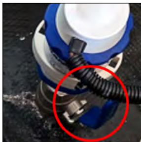
1100 GPH Fill Pump Valve Handle.
